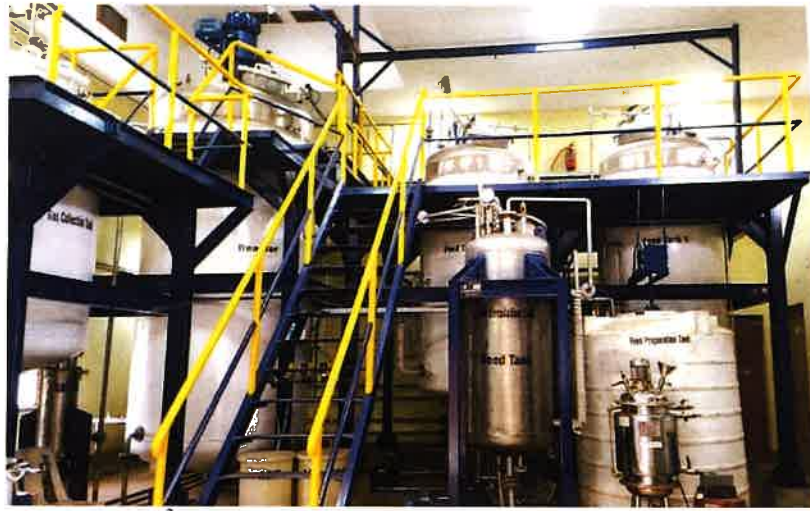
10 m 3 Biohydrogen Pilot Plant at IIT Kharagpur
