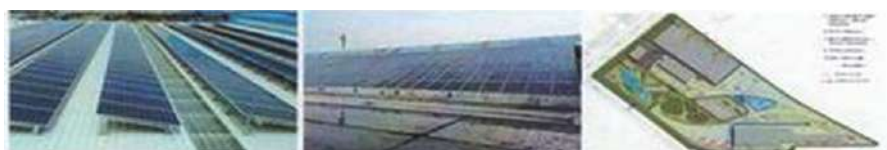
Rooftop Solar Power- Chennai Metro
